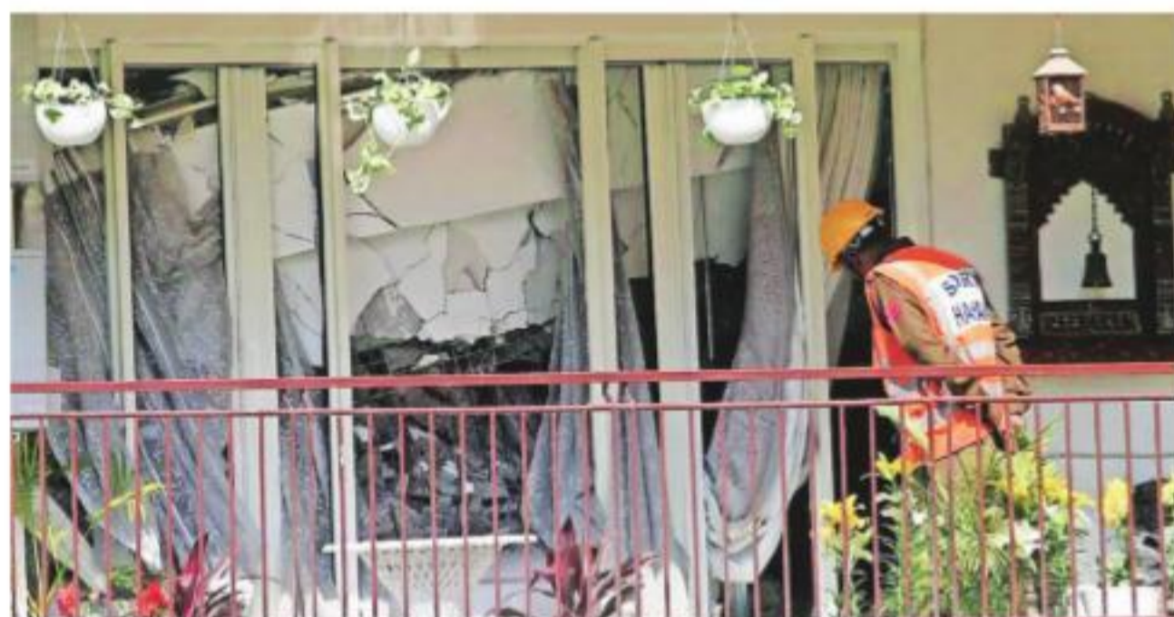
On Feb 10 last yr, a portion of a flat in Tower D collapsed, killing two women. Archive
