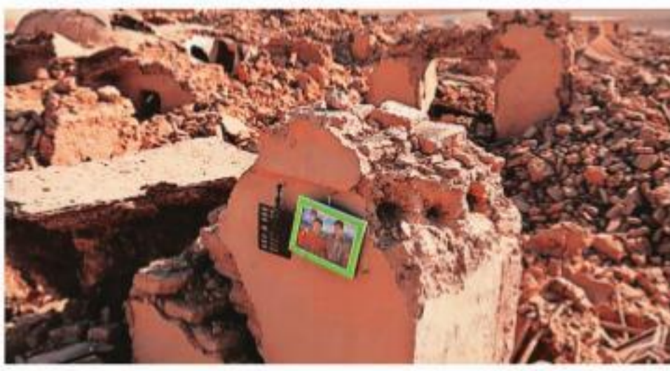
A family picture on a wall of a damaged house after earthquake in Herat province, West Afghanistan, Wednesday. Reuters
