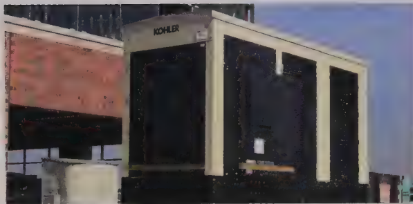
Generator types range from small portable units to large permanently installed, pad-mounted units with large fuel-driven engines.
