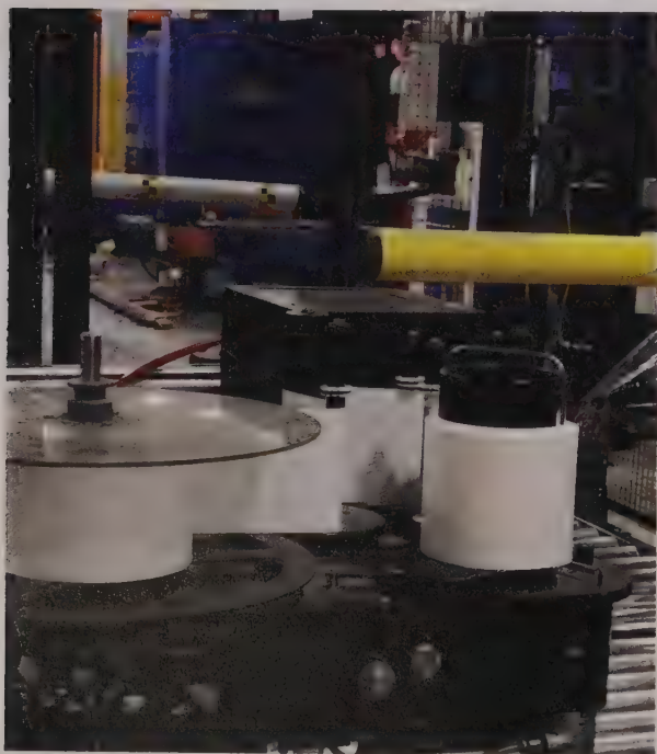
Machines used in commercial and industrial manufacturing and processing are time- and count-controlled by electrical and electronic circuits and systems.
