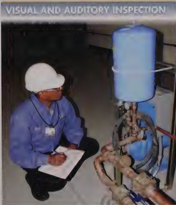
Figure 30-2. Maintenance technicians routinely check the appearance and sound of operating equipment using visual and auditory inspection.
