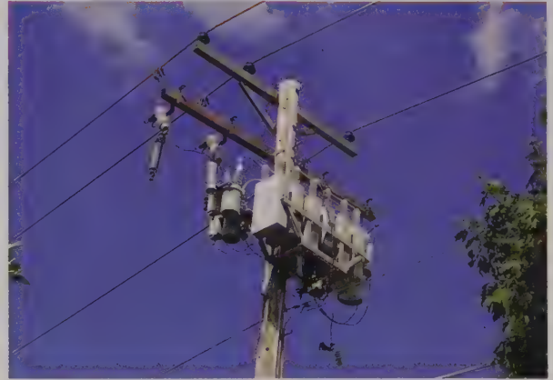
Distribution transformers are used to reduce high transmitted voltage to lower voltage levels that can be used for residential, commercial, and industrial applications.
