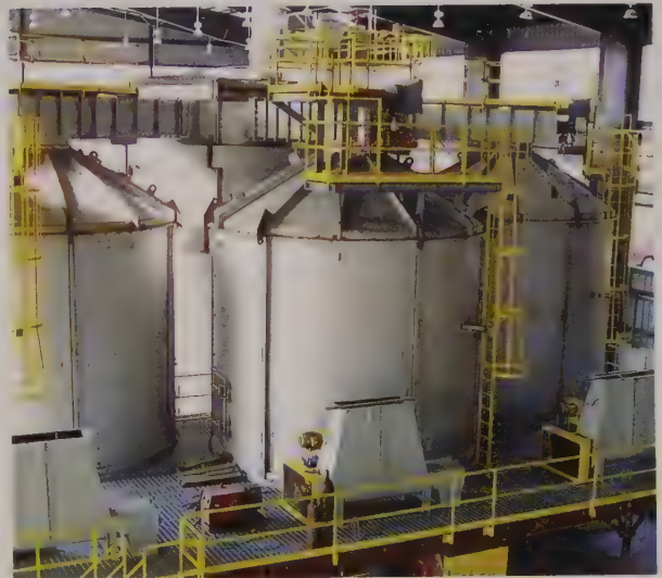
PACs can be used to control the fill of industrial-sized tanks.
