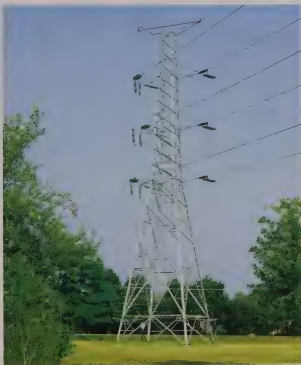
Transmission lines carry electrical power from distribution substations to step-down transformers.
