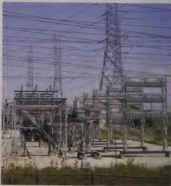
Distribution substations are located in close proximity to where the electrical service is provided.
