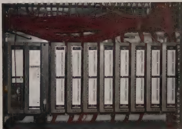
Programmable logic controllers (PLCs) and programmable logic relays (PLRs) have internal timers that must be programmed into a circuit.
