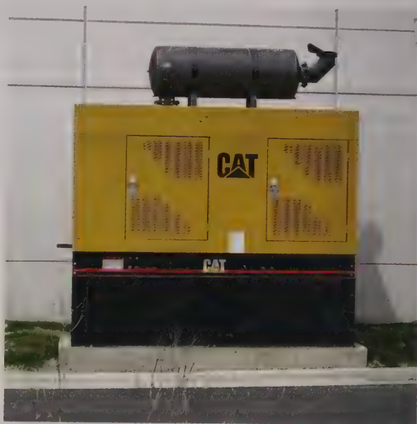
A generator is commonly used as an emergency power supply when the primary power supply fails.
