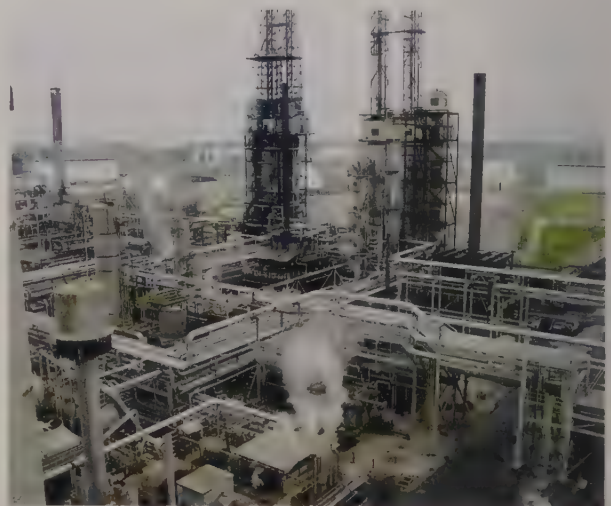
Programmable controllers are commonly used in large industrial facilities to control electric motors, valves, pneumatic or hydraulic cylinders, magnetic relays, and other devices.
