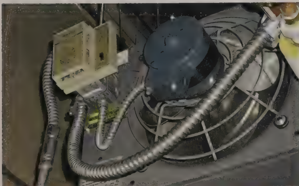
Fans used to cool equipment or circulate air are powered by motors.
