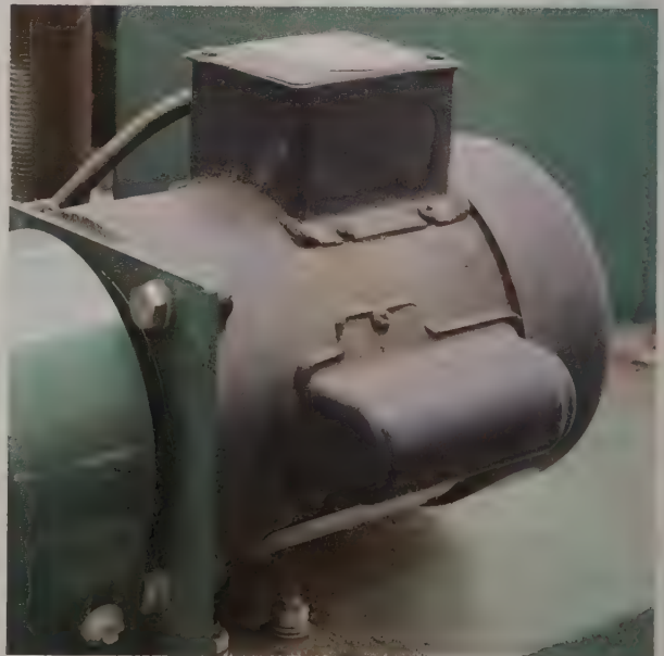
Equipment exposed to outdoor elements will require more frequent maintenance to prolong its life.
