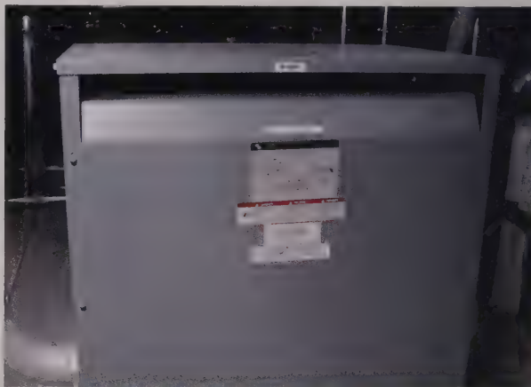
Taps on a transformer must be wired correctly to prevent overvoltages.
