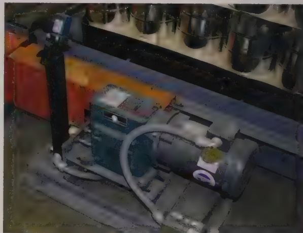
On-delay and off-delay timers can be used to control motors that operate conveyor lines.
