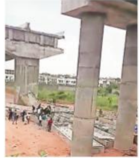
The collapse site. Express
