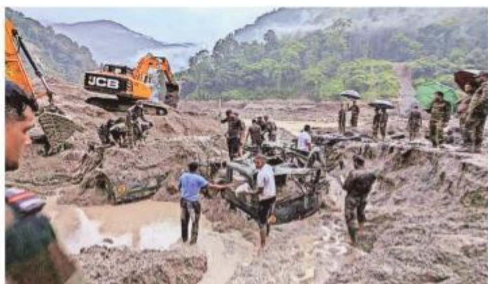
Army personnel try to recover trucks buried in a flood-hit area in Sikkim. Reuters
