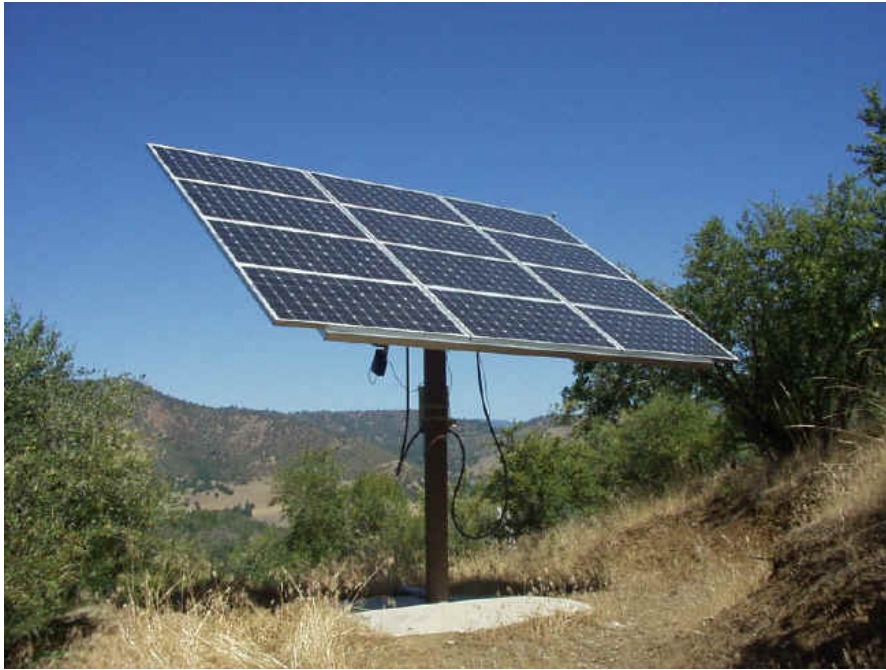
My Solar Panels Mounted on old C-band Satellite Dish Pole using Actuator Tracking.
