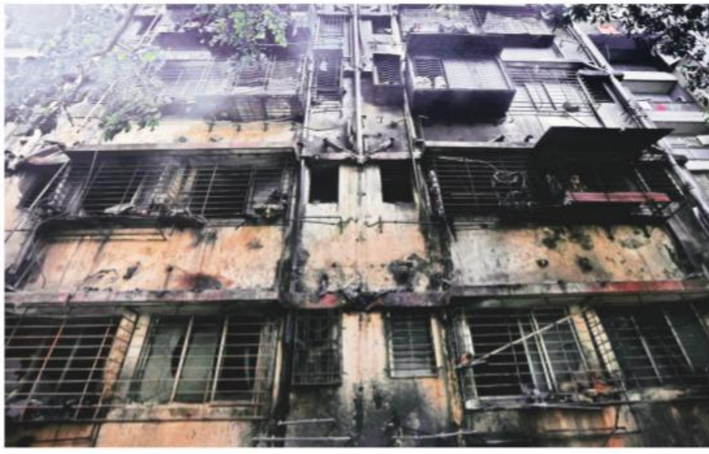
The fire broke out in a seven-storey residential building in Goregaon West. Amit Chakravarty
