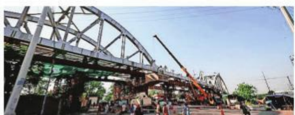
The under construction Rail bridge of Delhi-Meerut RRTS, over Kalyanpuri Chowk in New Delhi. Praveen Khanna
