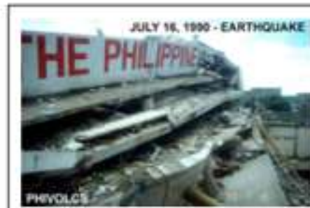
A school building in Cabanatuan City collapsed after intense ground shaking, trapping hundreds of students, 16 July 1990 Luzon Earthquake (Source: PHIVOLCS)
