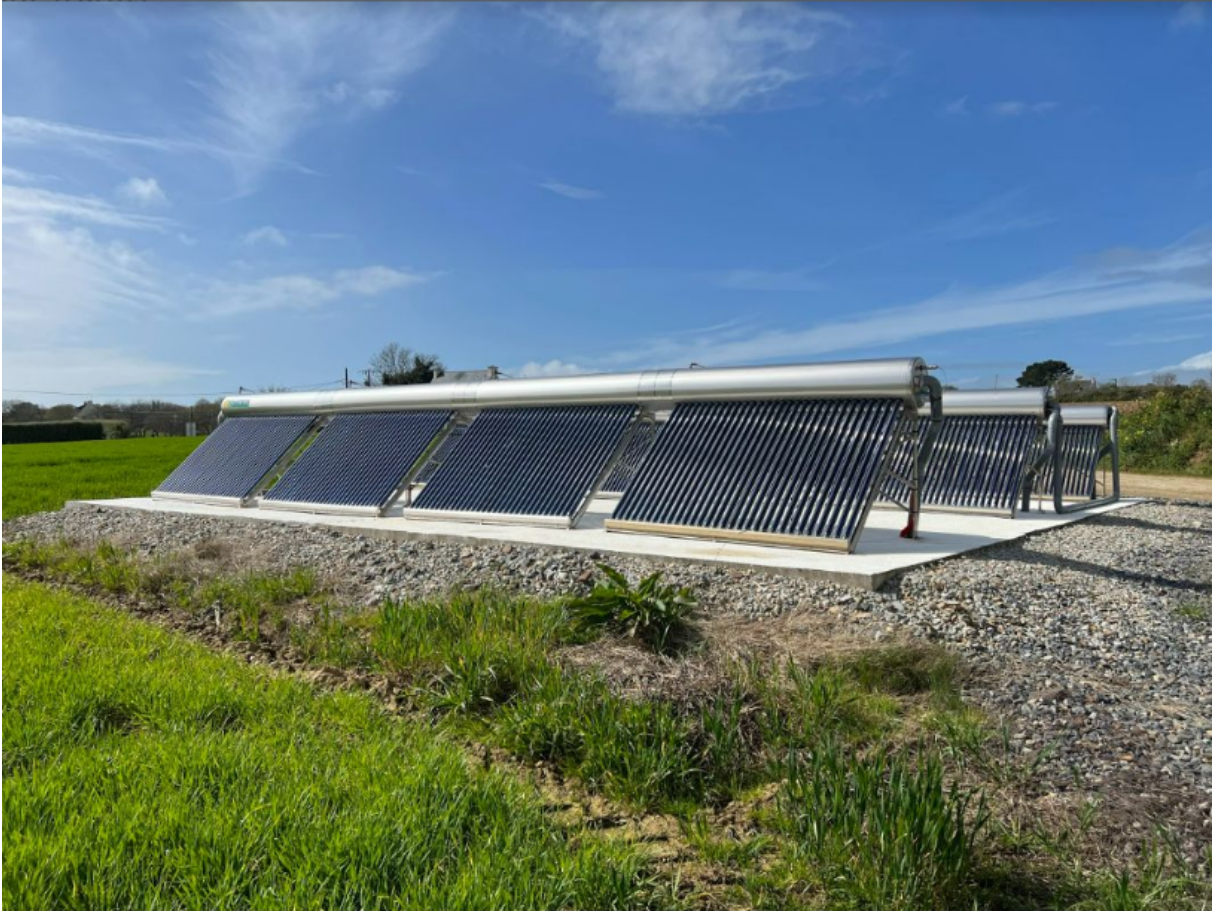
Figure 24: ICaRE4Farms STC installation, courtesy of the ICaRE4Farms LinkedIn page [1]
