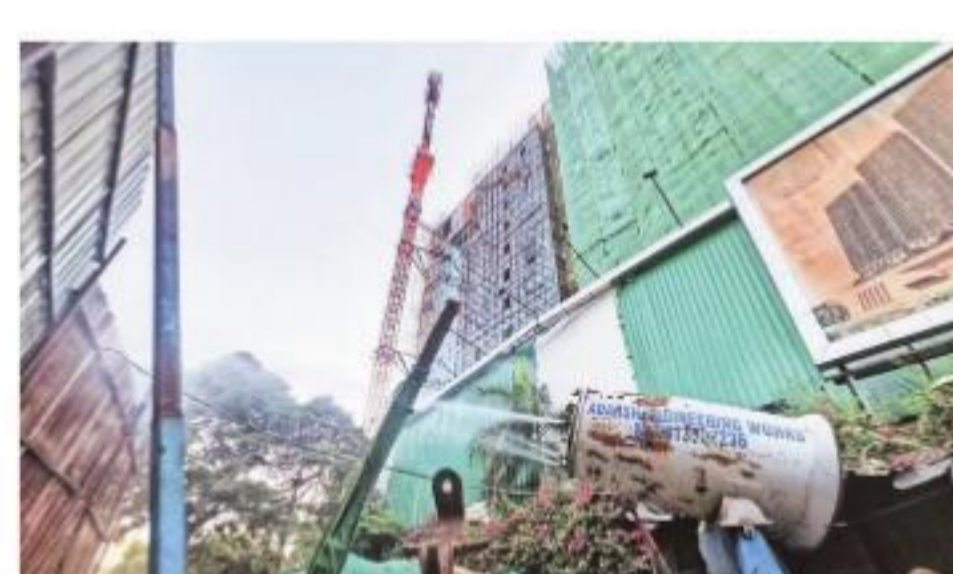
Smog guns have been mandated at construction sites as part of dust-mitigation measures. Abhinav Saha
