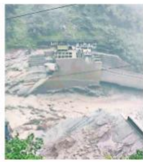
The Chungthang dam of the Sikkim Urja Ltd project was washed away on Oct 3. File
