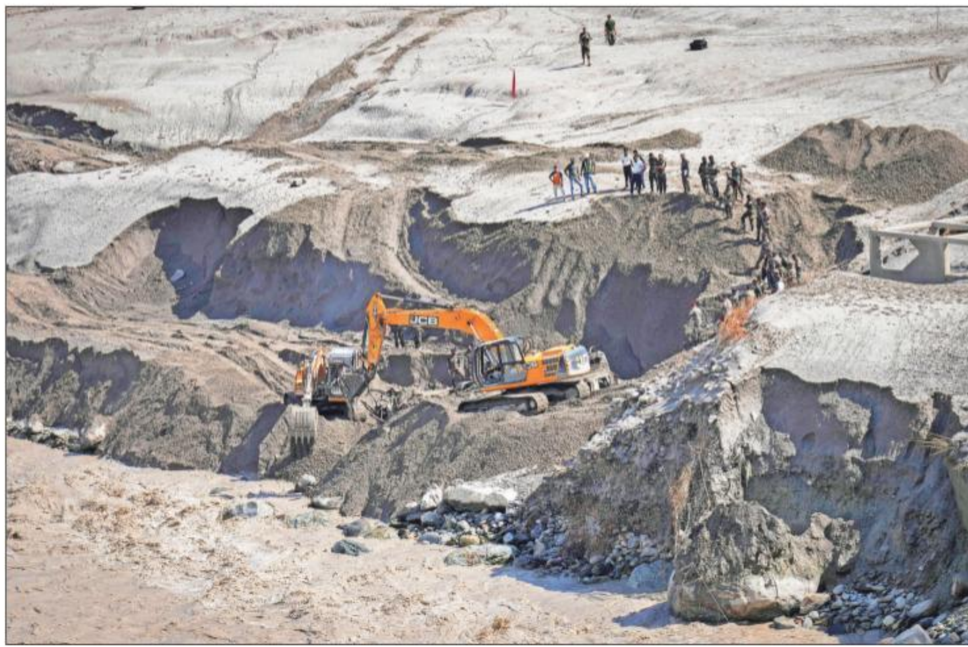
Army personnel dig along the Teesta as they look for missing people and vehicles in Sikkim's Bardang on Sunday. AP
