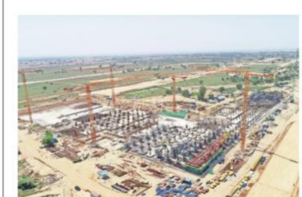
The site is strategically connected to NCR and Western Uttar Pradesh. Express
