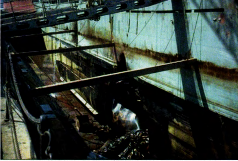
A view of the massive hole in dry dock
